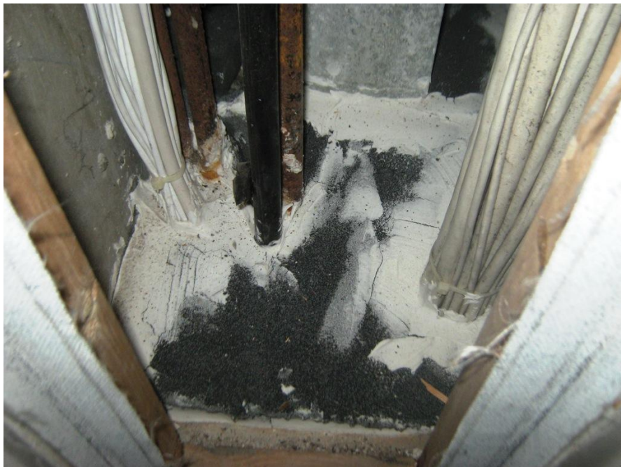
Photo 3 - Common area riser duct - Fire-stopping
