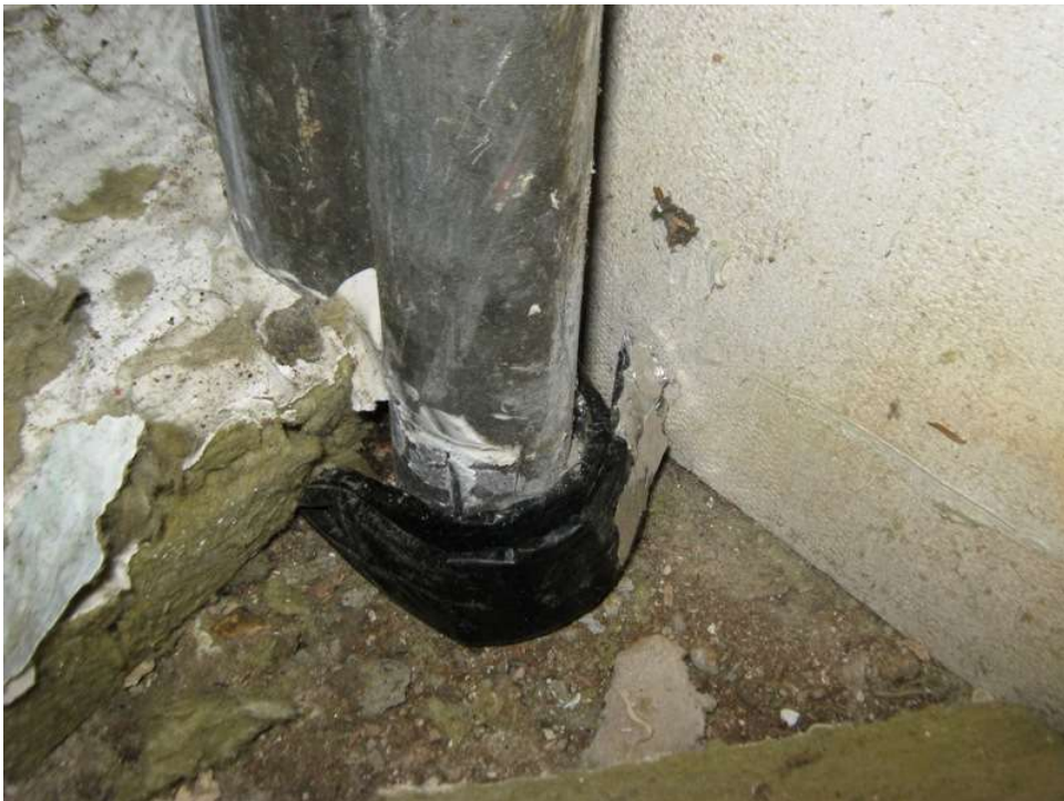
Photo 13 - Lower level duct – fire-stopping to floor slab.
