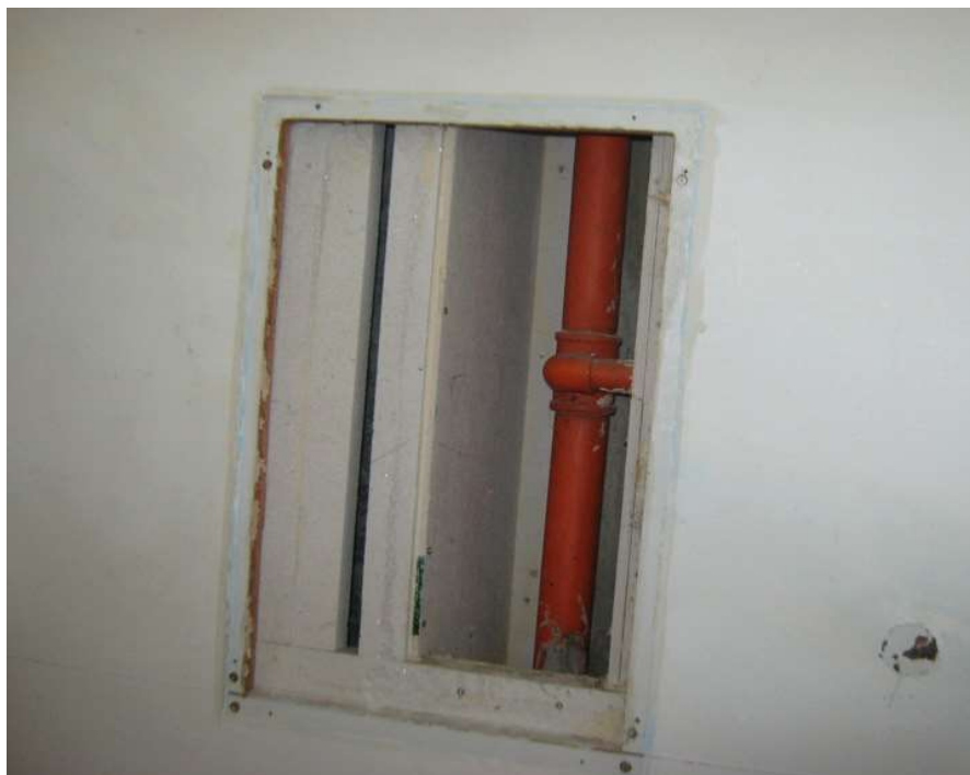
Photo 9 - Riser duct in apartment with access panel removed.
