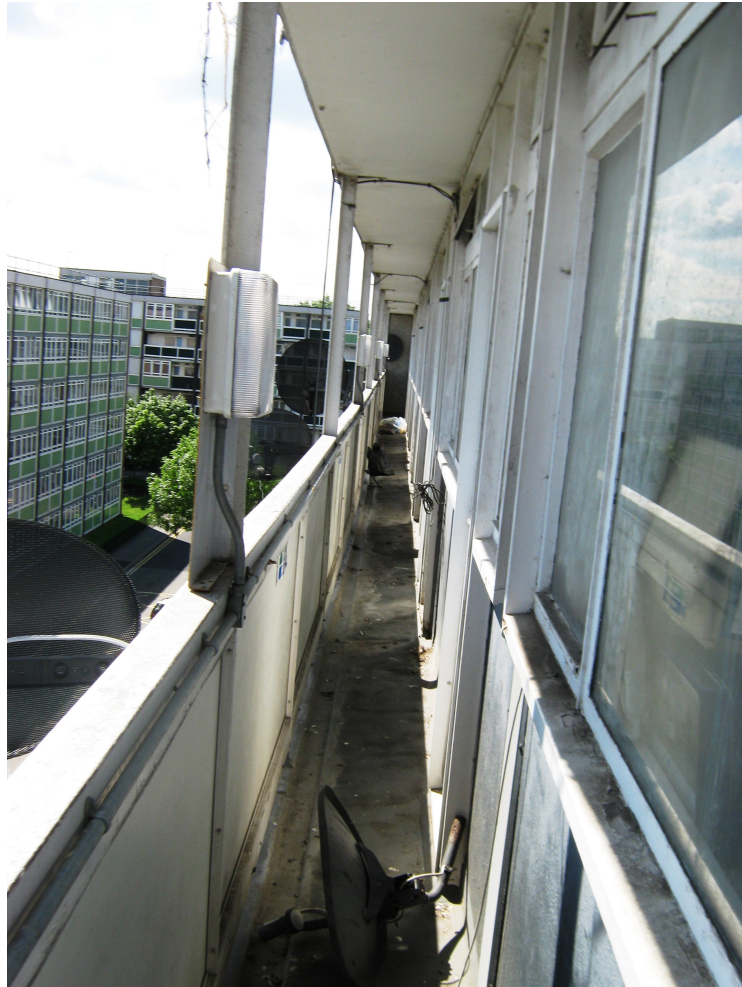
Photo 4 – Obstructions to emergency escape balcony.
