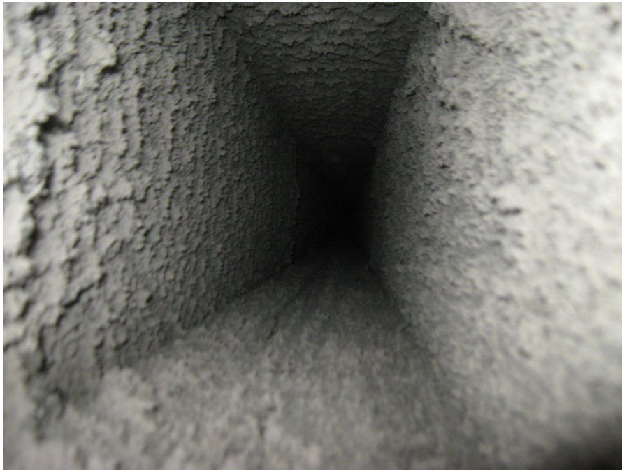
Photo 8 - Inside air extraction duct (note dust build-up).
