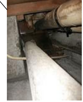
Cement boarding at pipe penetration point
