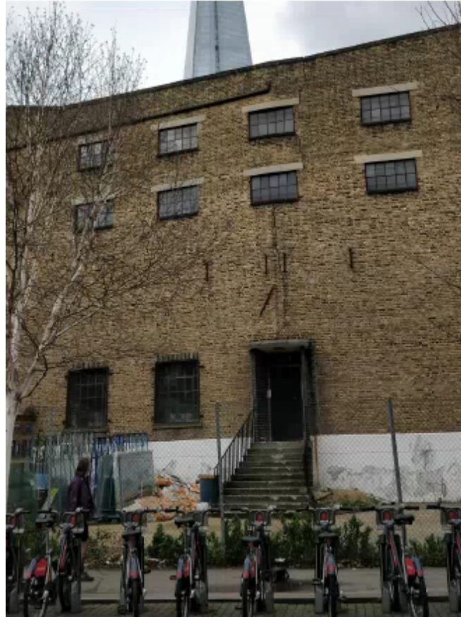
View of South wall from exterior showing vertical crack
